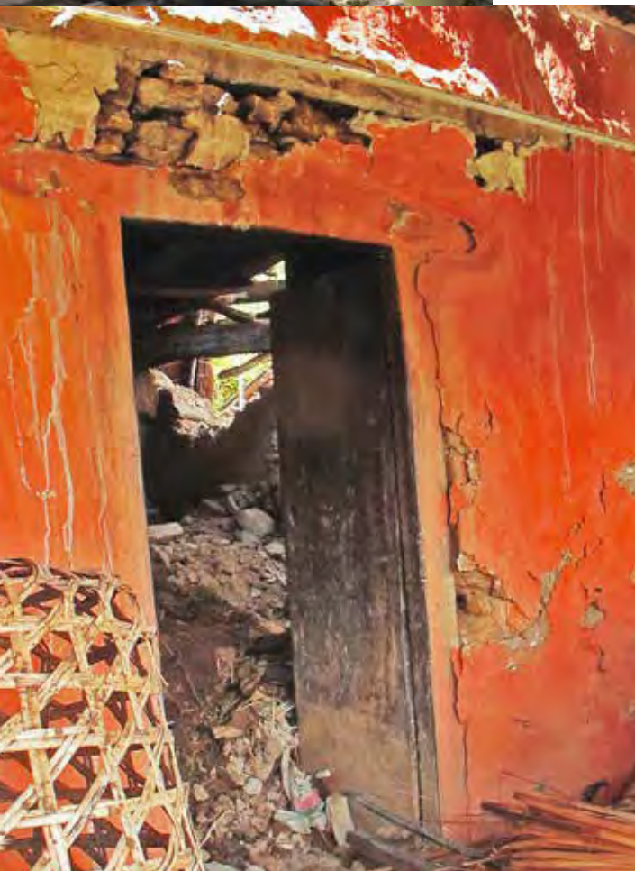
Top photo: A temporary shelter made of tin and tarps. Bottom: What is left of one family's home after the earthquake.
