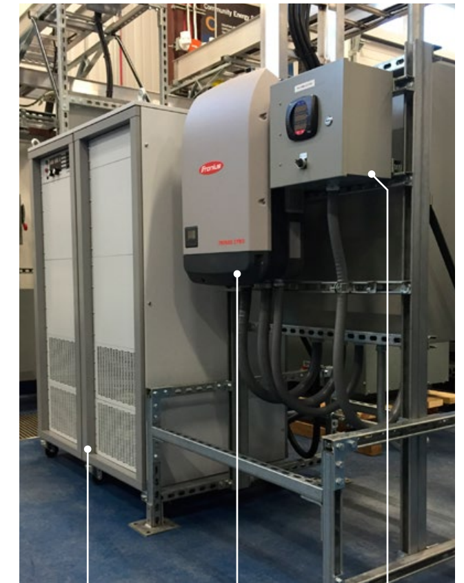
Magna Power DC power source Fronius inverter power meter
