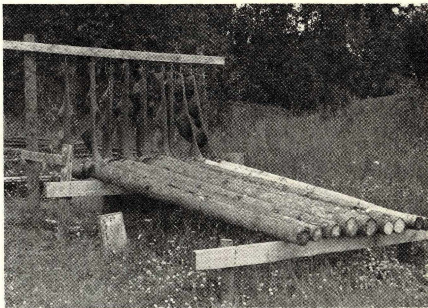
Poles supported in a rack for treating by the "fire-tube" method. Oil drum holds treating solution. Bucket and scales are for measuring chemicals.
