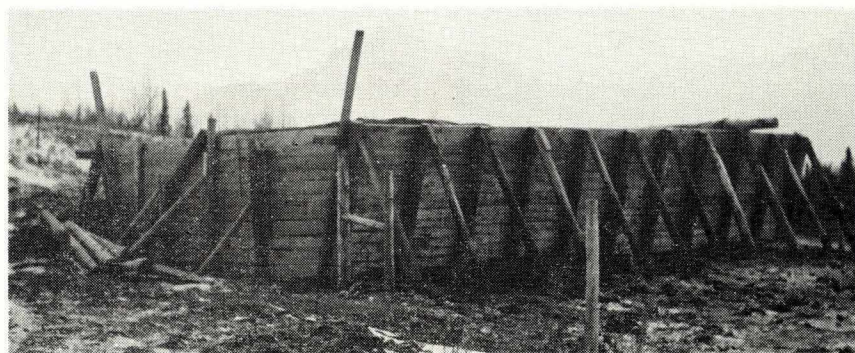
A sloping site insures good surface drainage away from the silo. Uniform slope and plenty of space at the ends gives a chance to extend the storage structure for future expansion.
