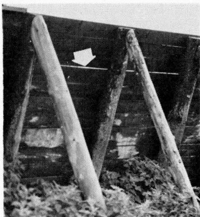
Green rough lumber shrinks to form wide cracks (arrow). Cracks are sealed by lining walls with plastic or moisture proof paper.
