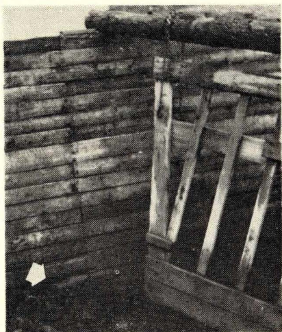
Arrow points to rotting boards at bottom of wall caused by excessive moisture. Muddy floor can be improved by pouring cement slab.
