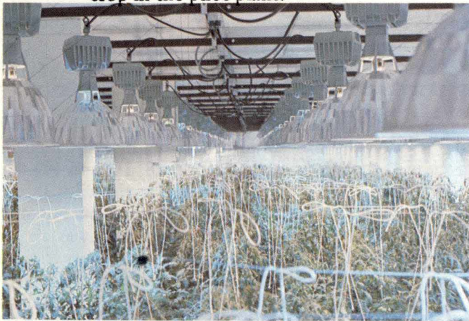
Figure 10: An overall panorama of the lighting in the pilot plant.
