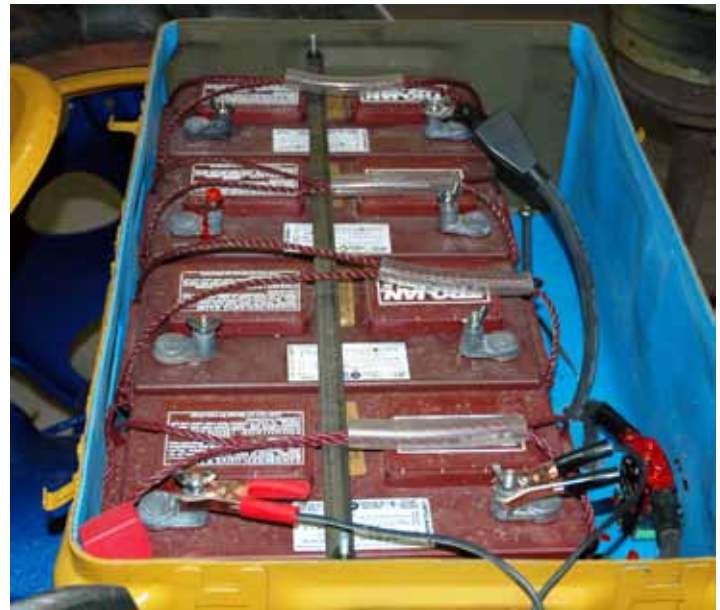
Photo E: Battery box holding four 12-volt batteries and miscellaneous other electrical components.
