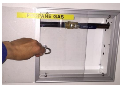
Figure 3. Removal of Plexiglass plate covering valve
