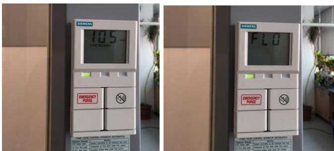
Figure 1. Fume hood monitors showing acceptable air flow readings.
