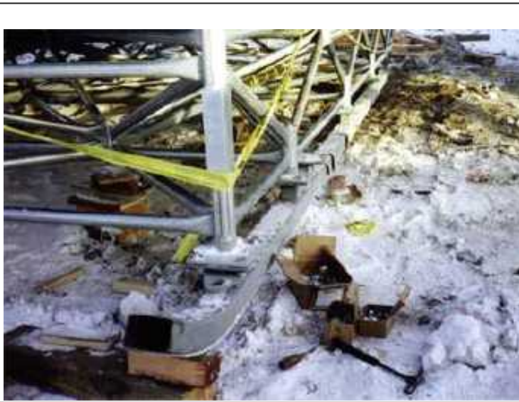
Photo 3: Close-up of the Ski Skid.
