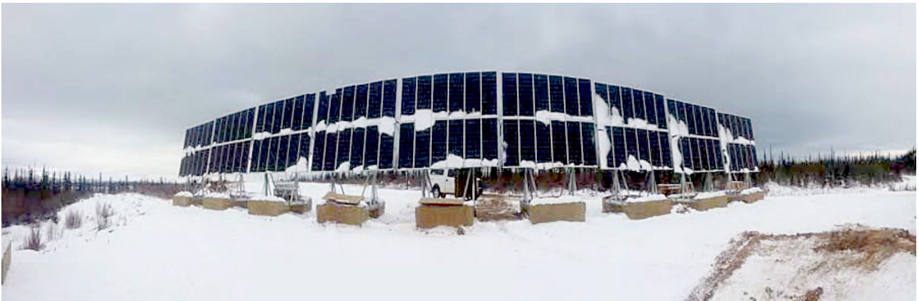
This wide angled picture shows the ballasted ground mounted solar PV array in Colville Lake. Photo courtesy Northwest Territories Power Corp
