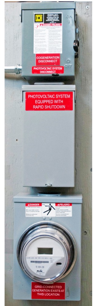
A disconnect like the one above is typically placed between the PV panels and the inverter.
