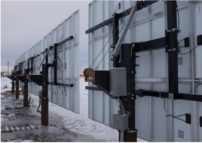
Figure 10. The manually adjustable pole-mounted PV array in Bethel is shown. Staff reportedly change the array tilt manually four times each year to maximize production and snow shedding. Photo by Chris Pike, ACEP
