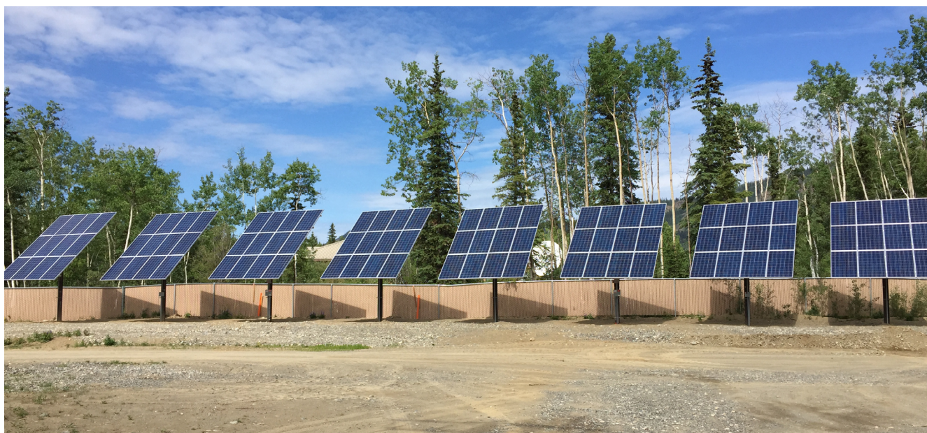
Pole mounted solar PV arrays in Eagle, Alaska (Photo courtesy Alaska Power and Telephone)
