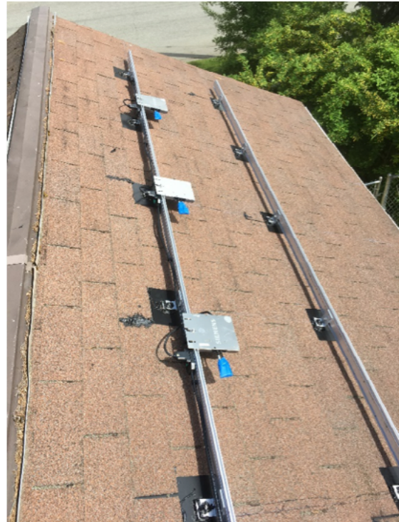
L bracket flashing, rails, microinverters and trunk cable
