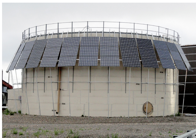
The circular PV array mounted on the water tank in Deering, Alaska. Photo courtesy Rob Bensin
