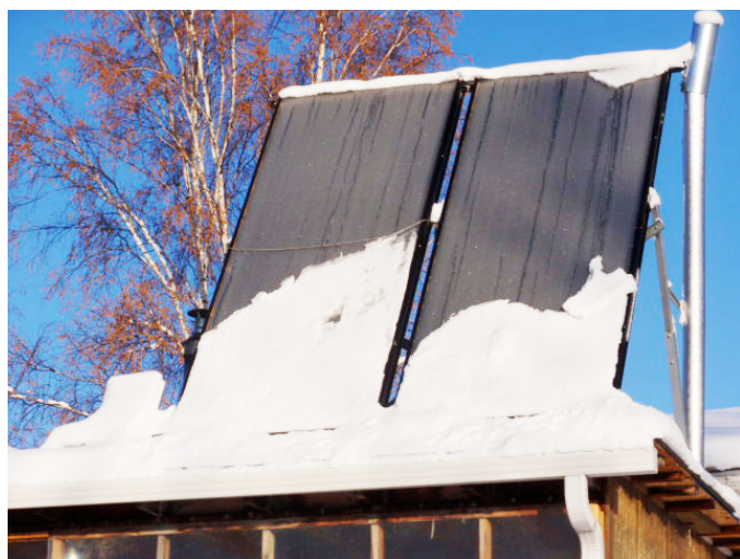
Figure 4. This photo shows the effects of the snow that is shed from the panel but accumulating on the roof, causing half of the collector to be blocked.
