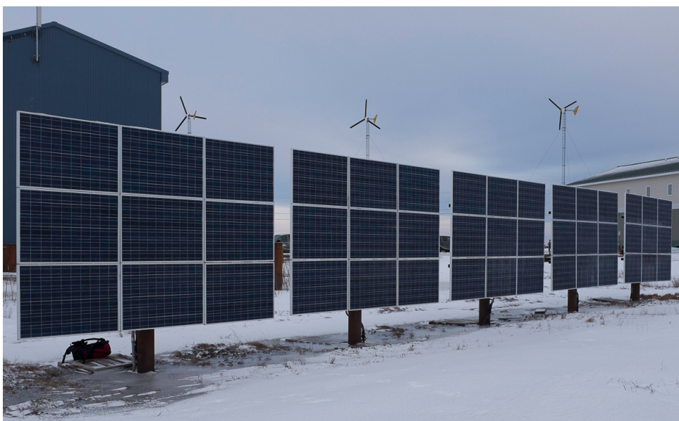
Figure 8. These pole-mounted PV arrays (left) located in Bethel are mounted on 8-inch pilings. In this photo they are facing south at a 90° slope. Photo by Chris Pike, ACEP
