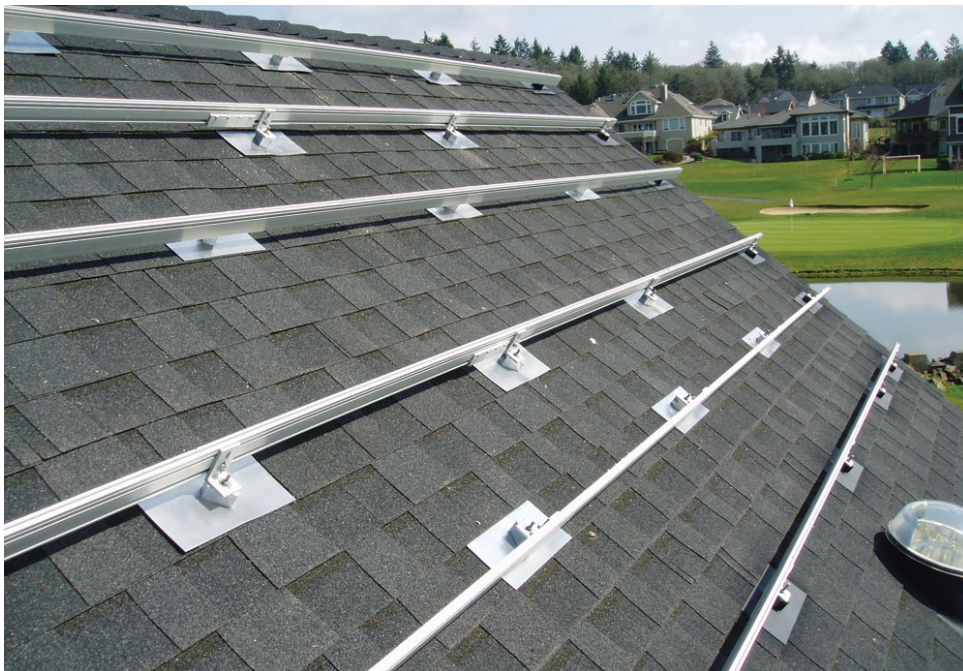
Figure 7. A roof-mounted racking system before the PV panels are installed. This system is mounted at the same slope as the roof. Courtesy quickmountpv.com
