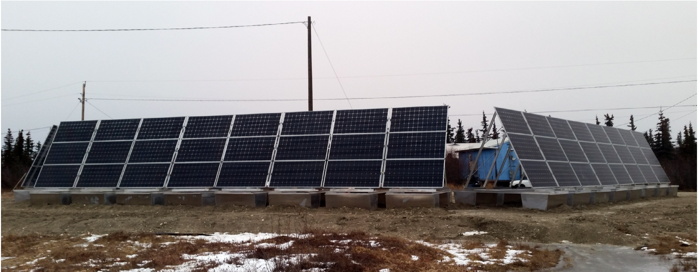
Figure 9. This ground-mounted array (below) is installed in the village of Noorvik in Northwest Alaska. The panels are oriented in three different directions to spread the solar production throughout the day and minimize the issues resulting from the integration of PV into a diesel microgrid. Photo courtesy Rob Bensin
