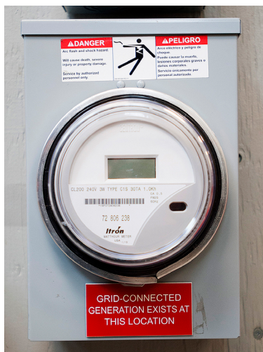
A typical kWh meter provided by the electric utility.
