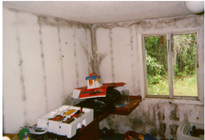
This photo shows several aspects of a house, which is poorly insulated at the studs — you see condensation and mold not only at the top of the wall where the wall plate is, but also in the corner and at each stud. This is an extreme example of a phenomenon called "ghosting of the studs" where the surface of the wall on the inside of the stud is cooler and therefore condenses out moisture and other vapors on the cool surface resulting in thermal bridging. Photo by Scott Waterman
