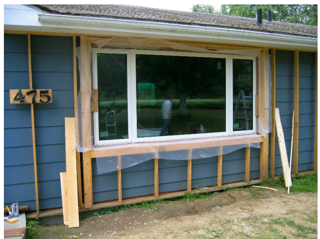
A house retrofit showing both the exterior wall being framed in and a new superinsulated window being installed in the rough opening of the old wall. Both of these are examples of how to retrofit both windows and walls with more insulation and a better performance window.
