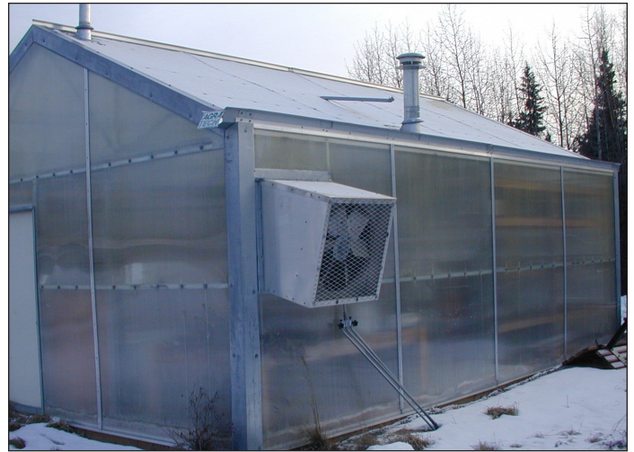
Picture 4. Freestanding greenhouses usually have fans at one end of the house and vents on the other.
