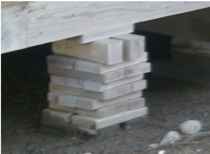
If your home is set up on crib timbers, they need to be connected with hardware to the structure.
