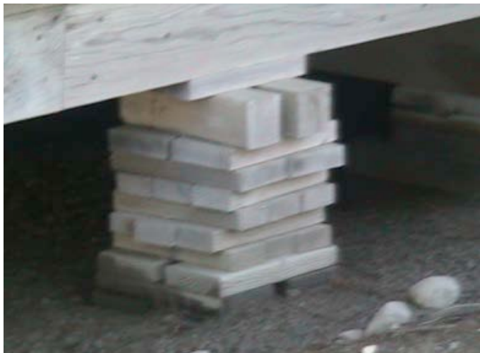
If your home is set up on crib timbers, they need to be connected with hardware to the structure.
