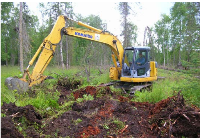
Mechanical site preparation is used to remove enough competing vegetation to enable successful tree seedling regeneration. Glen Holt photo
