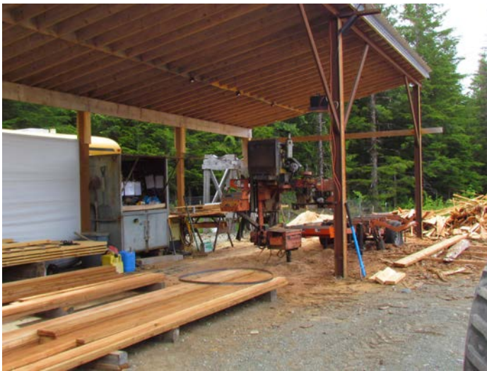
JK Forest Products has two sawmills. This is an LT-40 Wood Mizer band sawmill. Glen Holt photo
