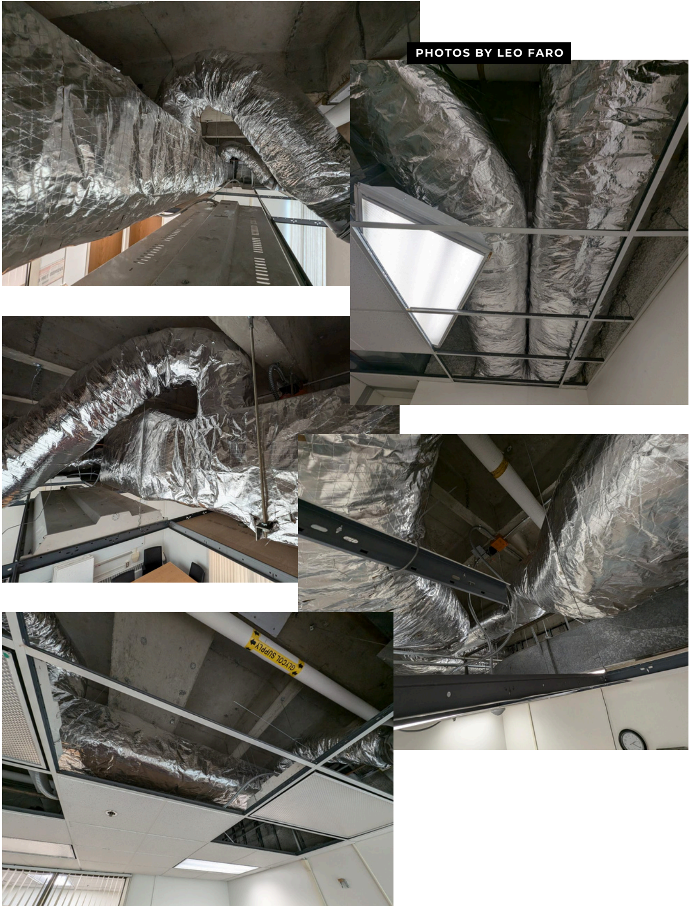
Some photos of the duct-work that was insulated the first two weeks of July during our insulation project. The work was done by Industrial Insulation Inc.
