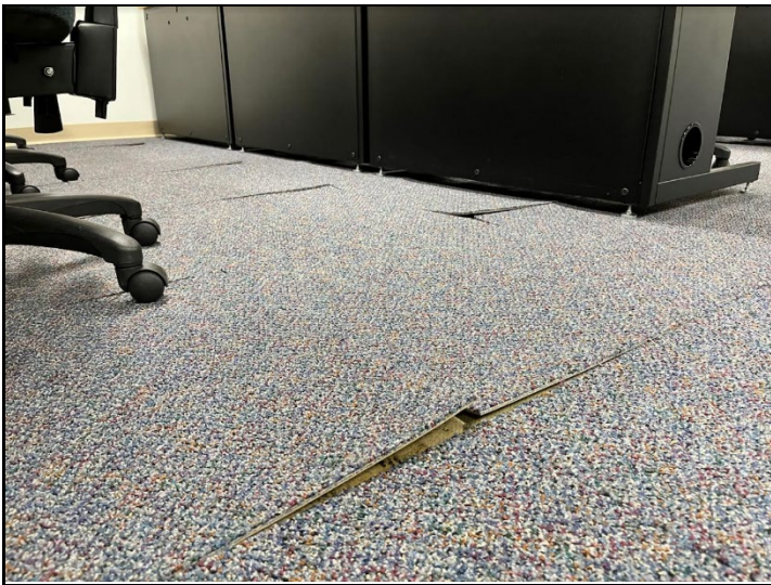
The tiles present an obvious tripping hazard.
