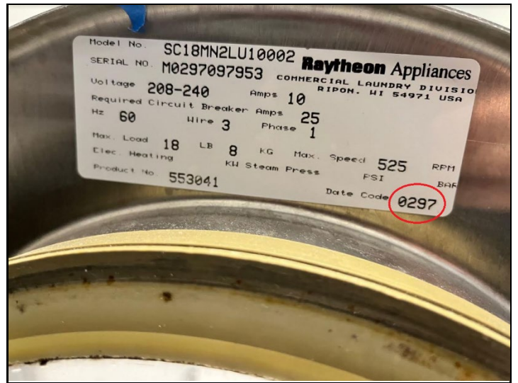
This Raytheon washing machine has been in continual service in Wickersham Hall since 1997, according to the date code on the appliance tag. It was installed as part of the building remodel that year, to meet ADA requirements for a wheelchair accessible laundry room. It's just amazing that this machine is 27 years old! Over its lifetime it's probably washed 50,000 loads of laundry.
