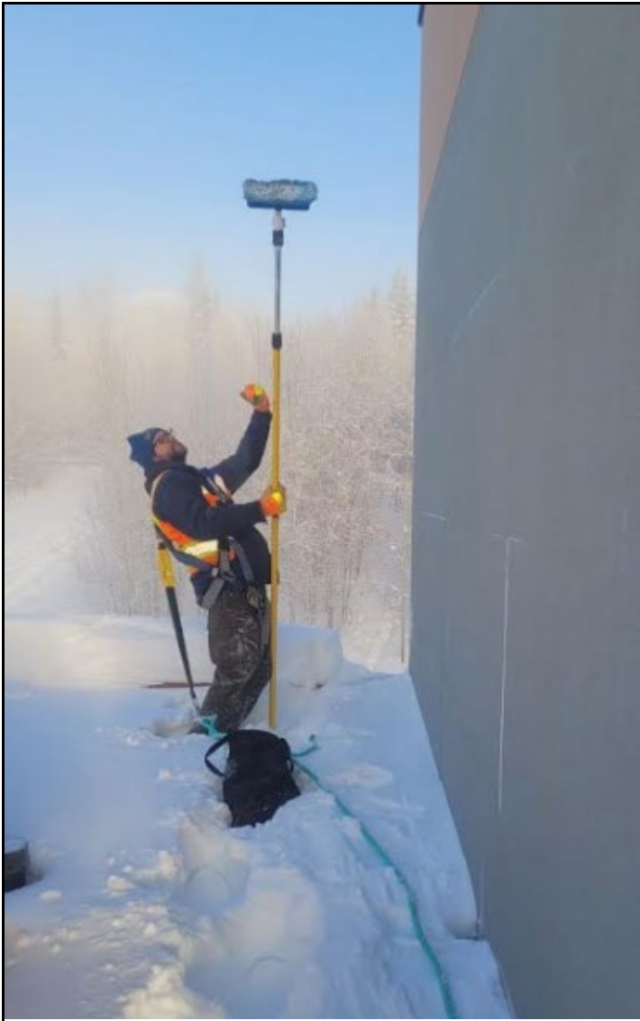
Ed Robinson from the HVAC shop had to climb out on the roof of Lathrop this past weekend to clear the ice buildup from the air intake. Nice job with the safety harness! Thanks to Thadd Williamson for the photo.
