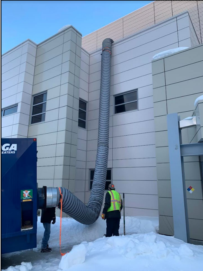
Our 1.5 million BTU Tioga heater was deployed to the BiRD building last Friday. In the photo above the hot air discharge hose is run up the side of the building and into the outside air intake. This setup kept the research animals inside the building comfortable during the steam outage.
