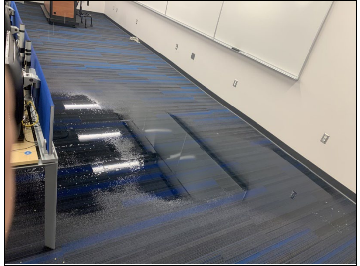
The computer lab in Duckering 530 was flooded by ethylene glycol because a seal failed on the cooling loop pumps in the penthouse mechanical room. Ethylene is considered hazardous material, so it needs to be handled with care. All the glycol was extracted from the carpet quickly, but the carpentry shop will still be replacing a large section of this flooring during Spring Break. Side note: The ethylene glycol in the district loop is colored blue so it can easily be recognized. Propylene glycol, which is far less toxic and used in most heating applications on campus, is colored yellow for the same reason.
