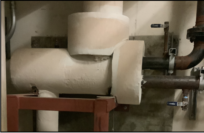
The shell and tube heat exchanger that provides heat for the UAF pool
