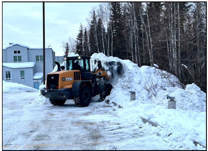
Unfortunately, we had to demolish the structure. The above picture shows Terry Beasley from Operations filling it in with the loader.
